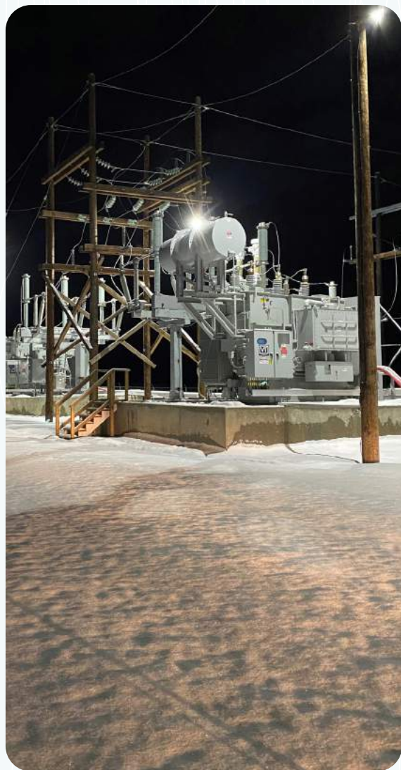
Victoria Gold sub-station.
